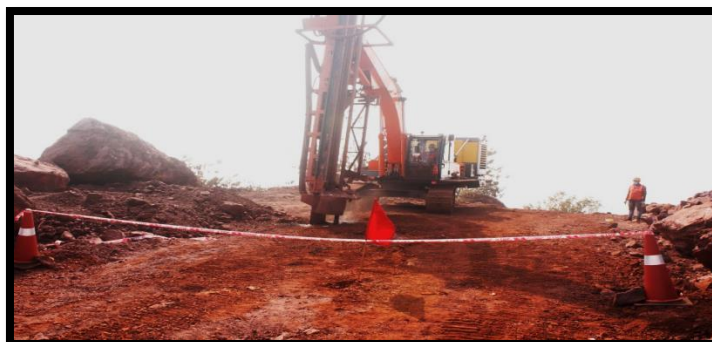
Photo Showing Excavate mounted Drilling Machine equipped with dust extractor & wet drilling mechanism
