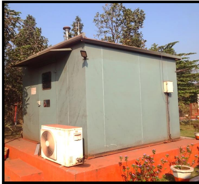
Photo showing the CAAQMS machine installed at mines
