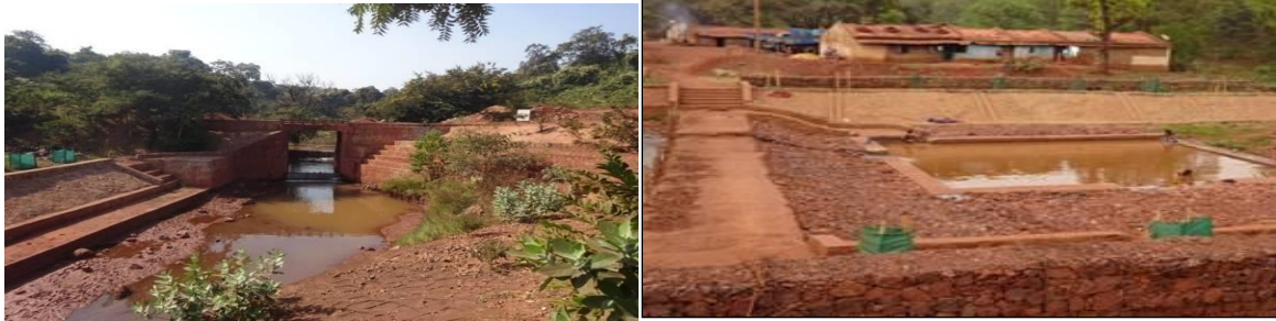
Photo Showing various Nallah protection measures undertaken outside ML
