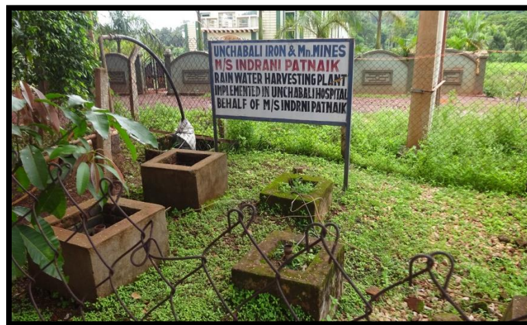
PHOTO SHOWING ROOFTOP RAINWATER HARVESTING SYSTEMS UNCHABALI DISPENSARY
